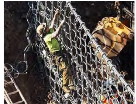
Figure 18: Debris Nets being installed in the upper canyons of drainage in the area.
